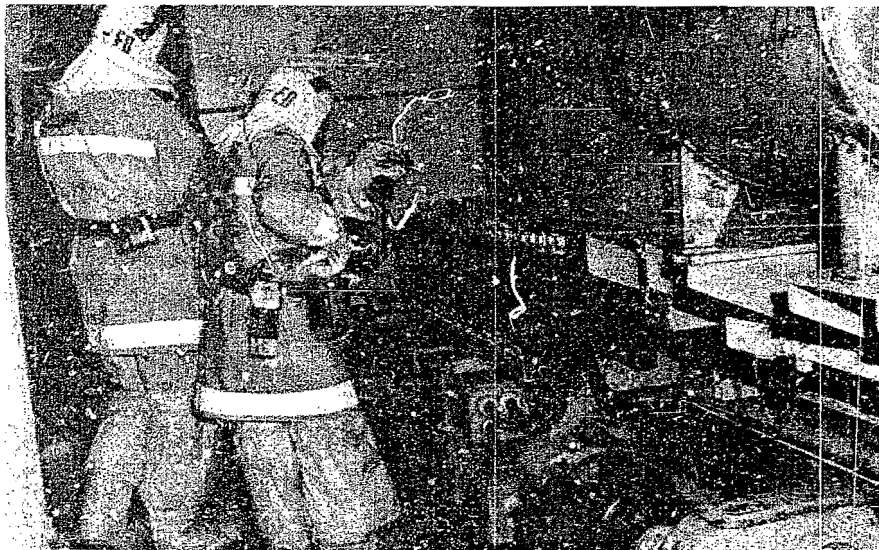
The entry team discovered extensive rusting on all of the metal around the power track.
